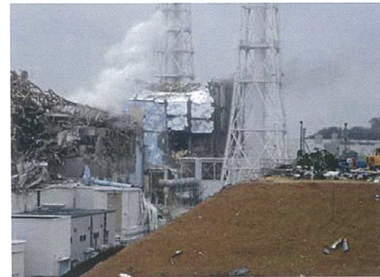
Fukushima Daiichi Nuclear Power Plant’s Unit 4, damaged by an explosion after the 2011 earthquake and tsunami.
